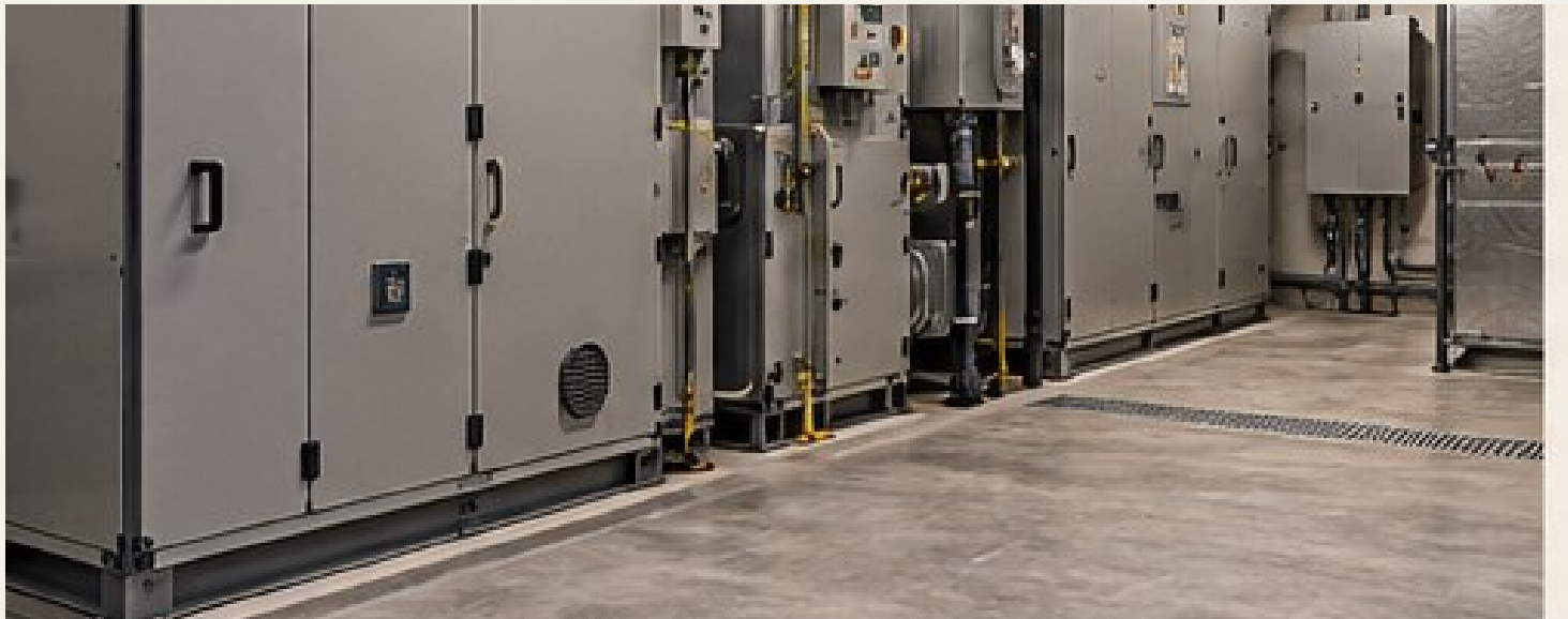
Dedicated air handling
